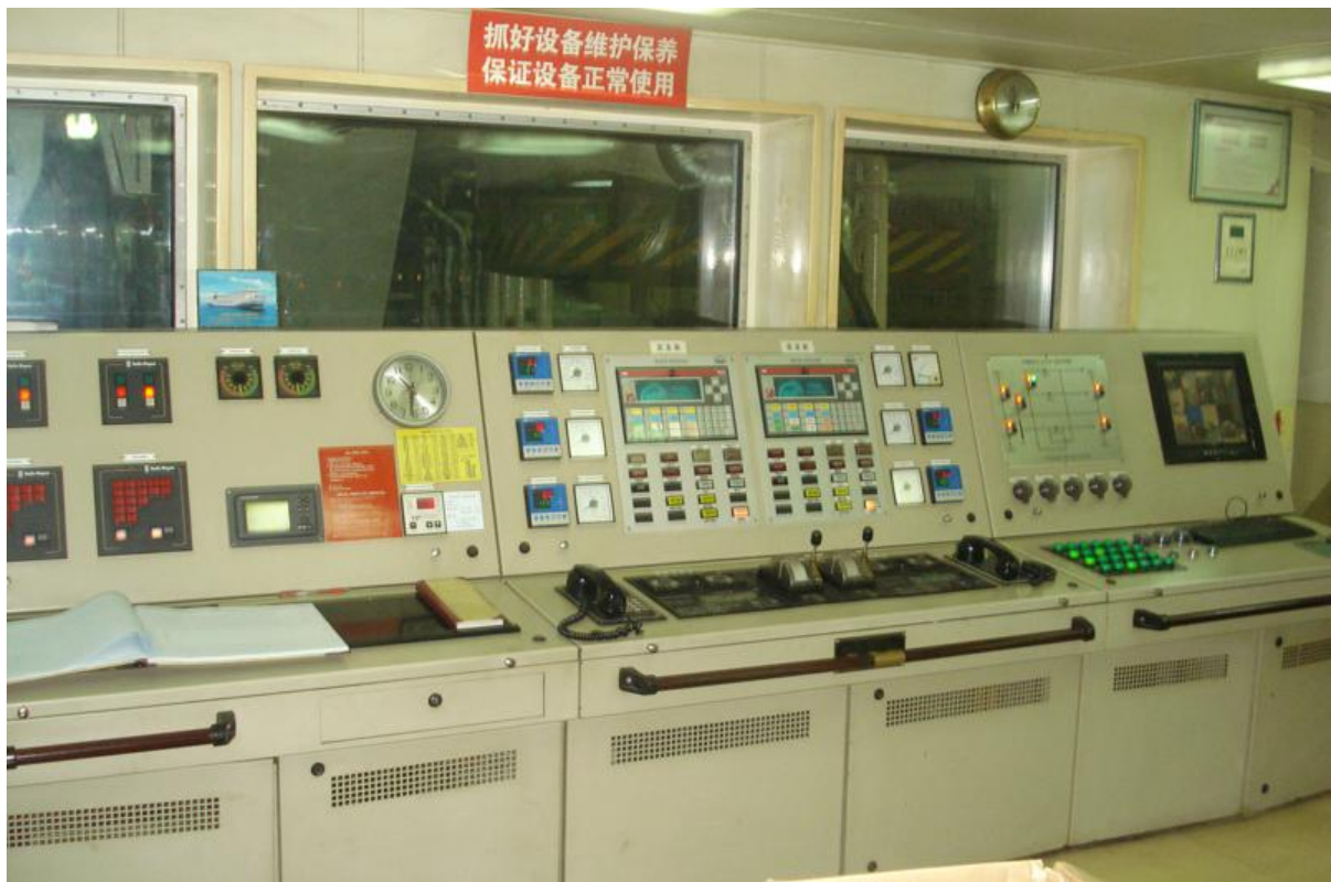
Engine Control Room
