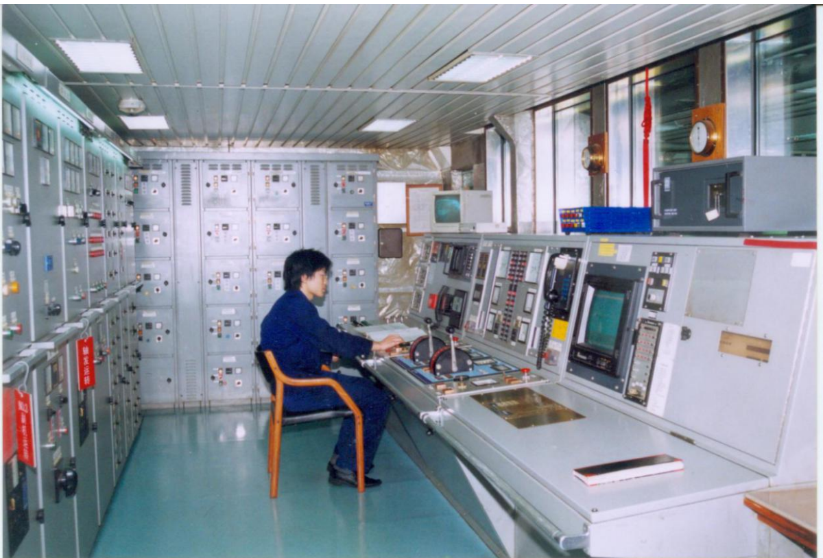
Engine Control Room
